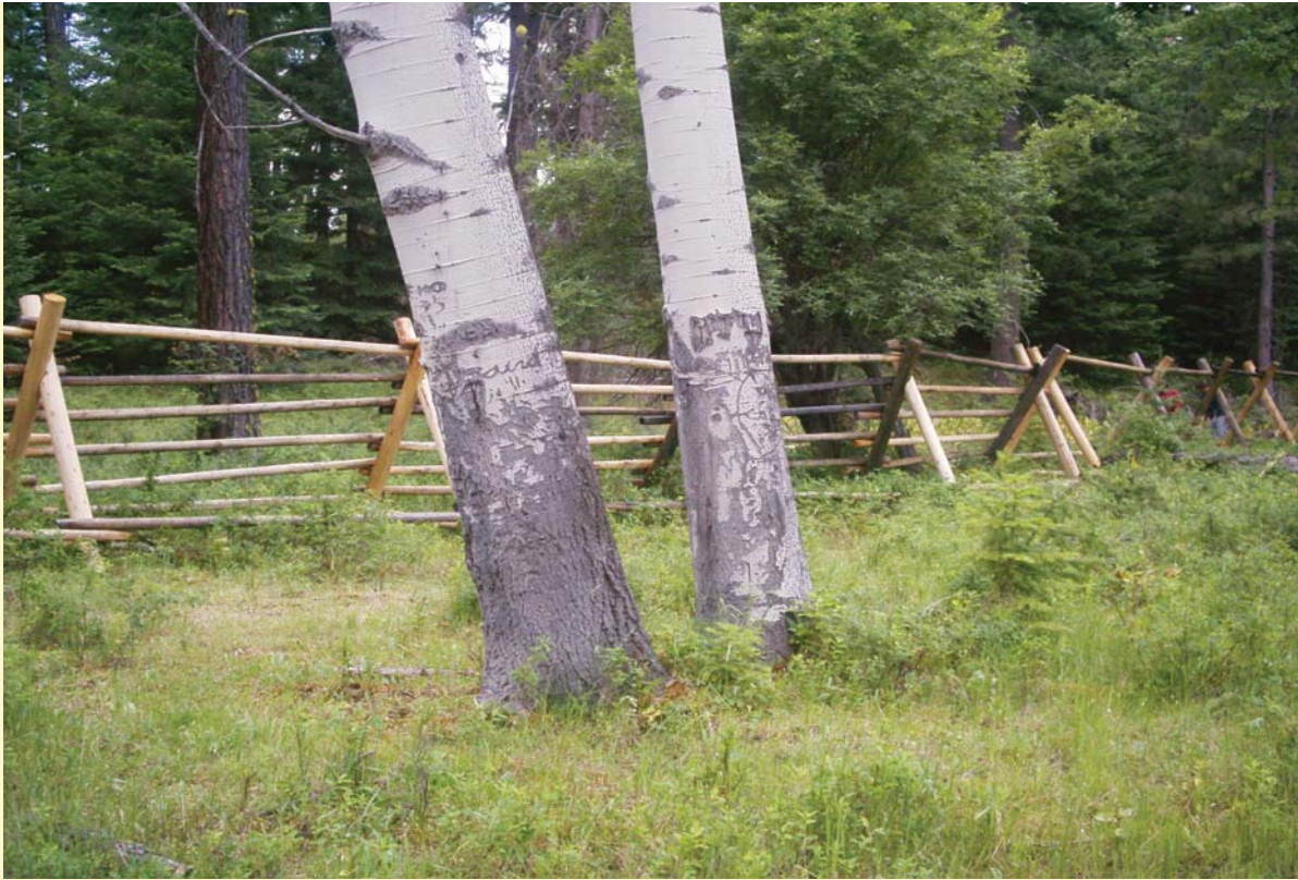
Interior of the fenced area with 9 th completed buck, Kevin and Aiden distributing rails, left, a pair of the mature aspen, a fir tree and an exceptionally clear, walkable space uncharacteristic of the terrain.
