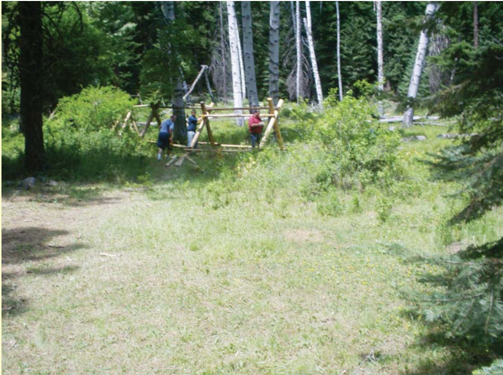
High rail being placed on a standing bucks. The standing buck has three rails attached, 1 high and two low. Four more are added close enough to keep juvenile elk out of the fence.
